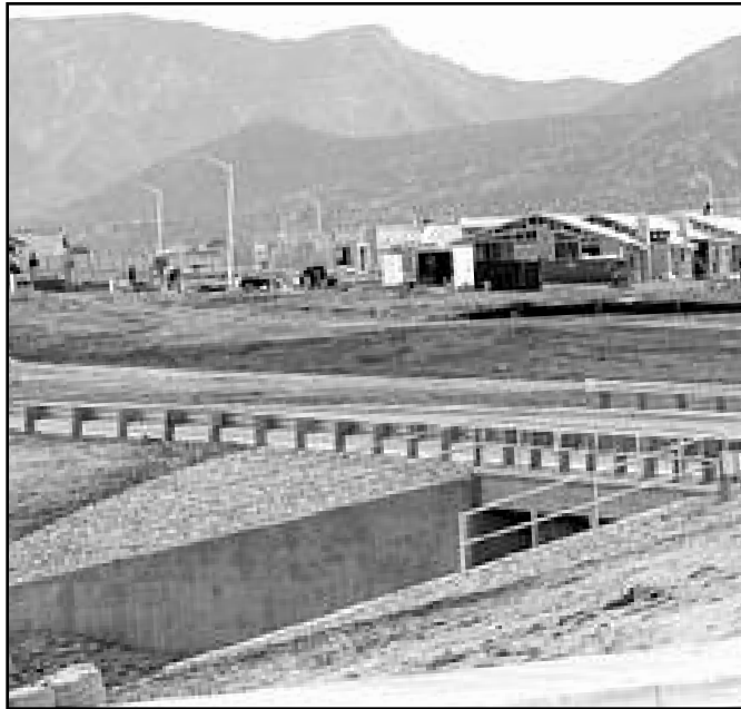
The St. Andrews Bridge may be finally getting ready for traffic as delays have kept the roadway from being utilized. Photo: Ed Honda-Herald/Review
