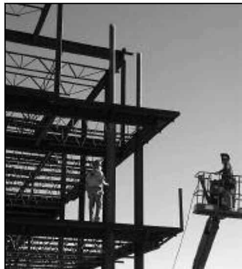
Construction continues on the new hotels located just outside the main gate to Ft. Huachuca. Photo courtesy of Sierra Vista Economic Development Foundation.
